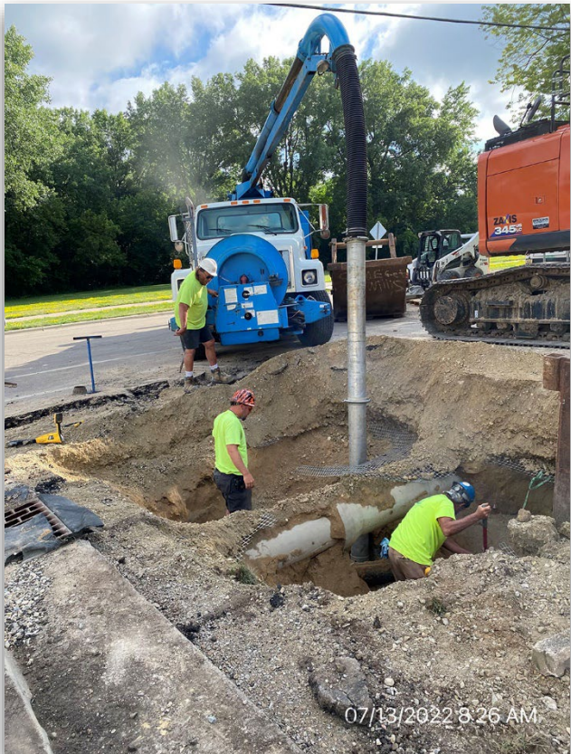
FOREST CONSTRUCTION WORKS TO COMPLETE THE CITY'S WATERMAIN REPLACEMENT PROJECT THIS SUMMER.
