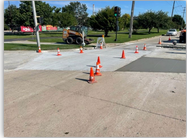
THE DEPARTMENT OF PUBLIC WORKS REPAIRED THE ROADWAY ON JANESVILLE AVE. THIS SUMMER DURING THE ROBERT STREET BRIDGE RECONSTRUCTION PROJECT.
