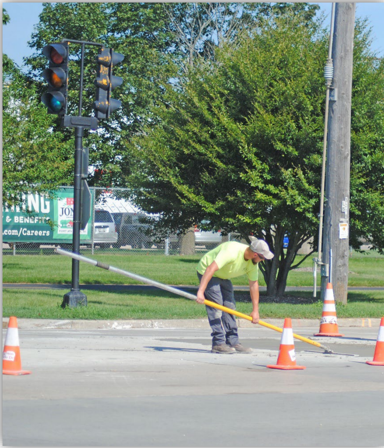
A MEMBER OF THE DEPARTMENT OF PUBLIC WORKS PUTS THE FINISHING TOUCHES ON ROAD WORK ALONG JANESVILLE AVENUE THIS SUMMER.
