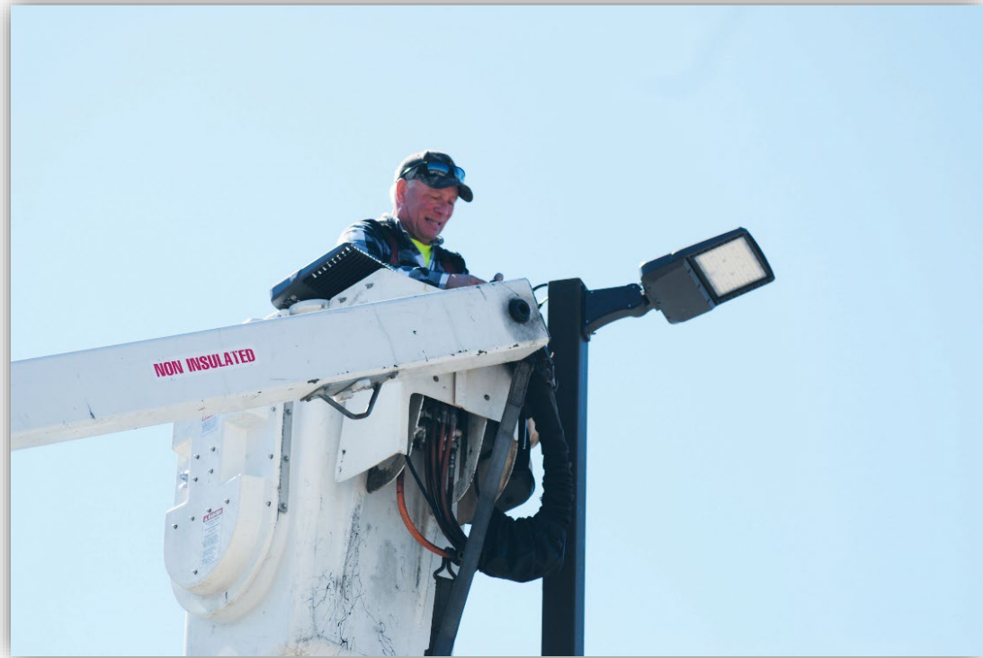
JEFF ARMSTRONG COMPLETES REPLACEMENT OF LED LIGHTS IN BETWEEN THE POLICE AND FIRE STATIONS.
