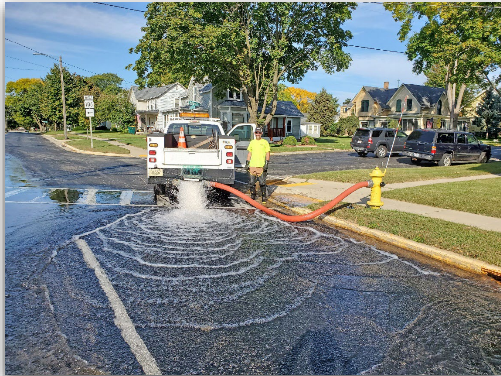
DAN SCHOENLEBER FLUSHES HYDRANTS IN OCTOBER AT THE CORNER OF ADAMS ST. AND SHERMAN AVE. W.
